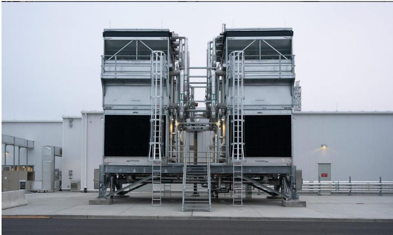
Outside air for direct free cooling.
