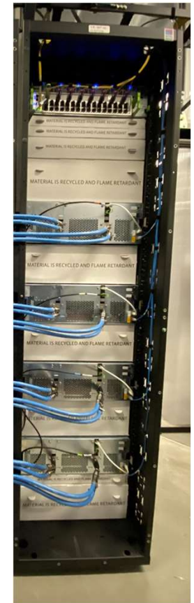
L11 rack and associated servers acquired from META for COOLERCHIPS project period.
