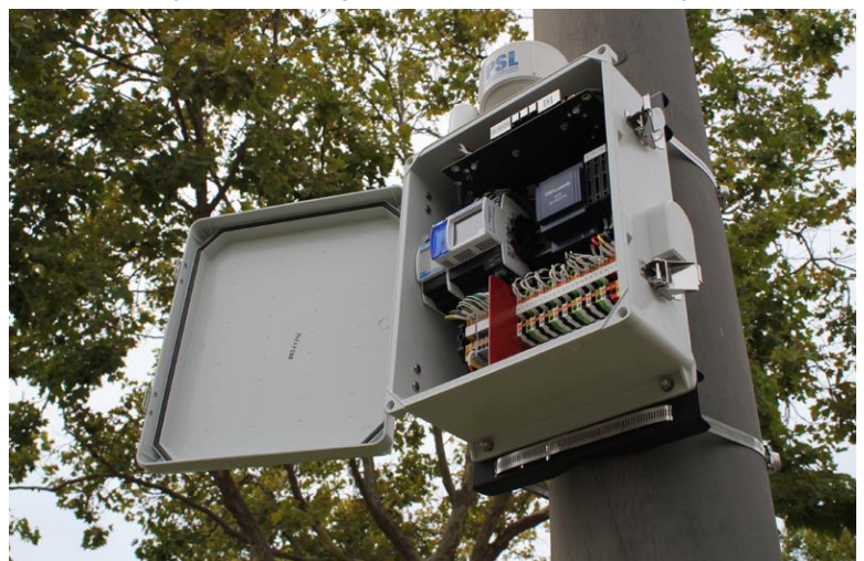
Figure 2: A \mu PMU installed on a utility electric distribution pole. The device consists of a high resolution power quality monitor and a GPS antenna (mounted on top of the box in this installation).
