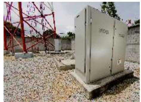
Figure 1: Fluidic unit installed in Honduras
